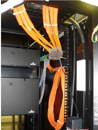
Single-mode sensing fibers in the cables that go from the PON splitter to the various ONU
