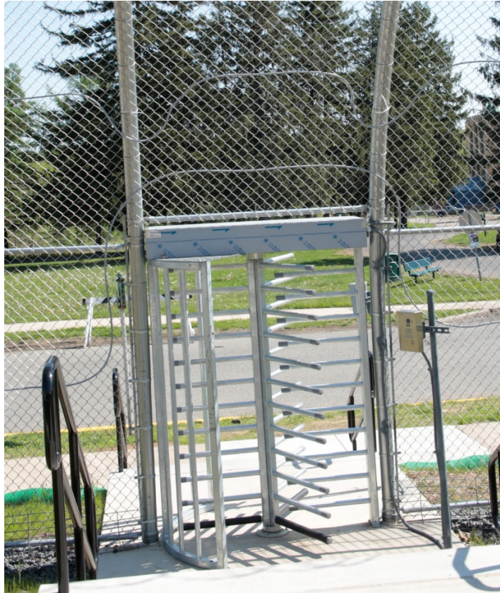
Figure 7. Turnstile personnel gate. The fiber runs up and over the gate and the gate is isolated from the fence system so that the vibrations do not cause unnecessary nuisance alarms from use.
