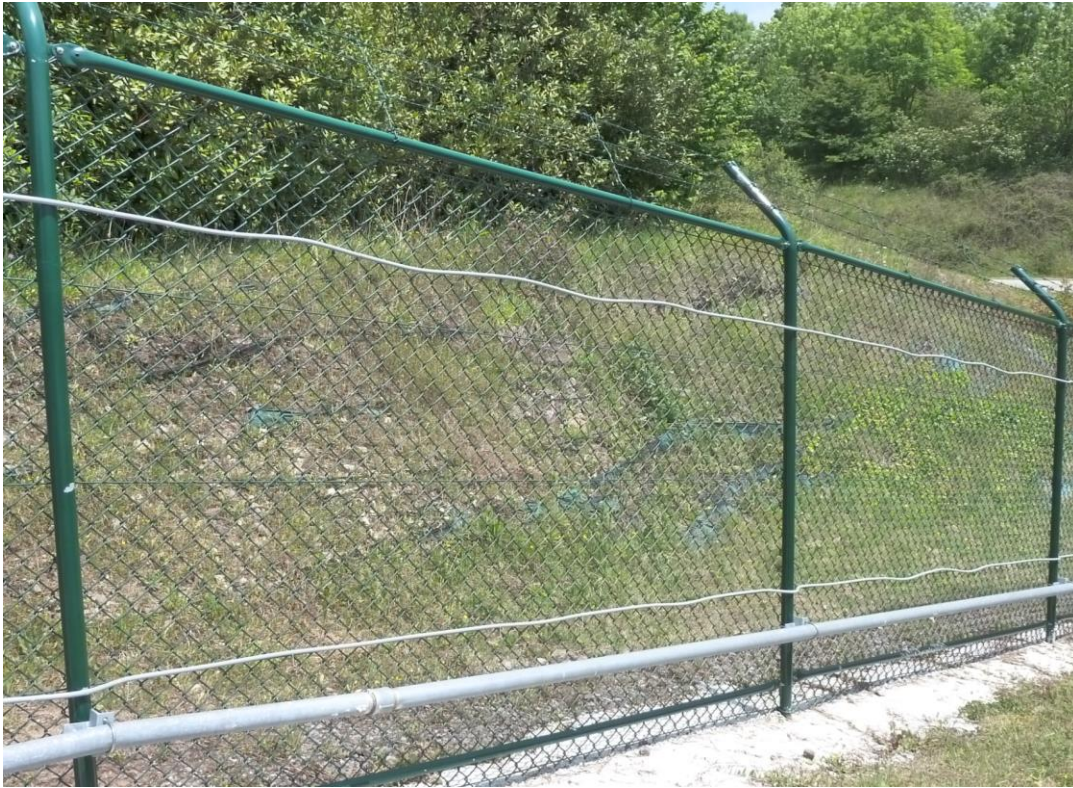
Figure 23: Observe the slight bend in the conduit due to hot and cold expansion; more ties and higher tension would prevent this phenomenon
