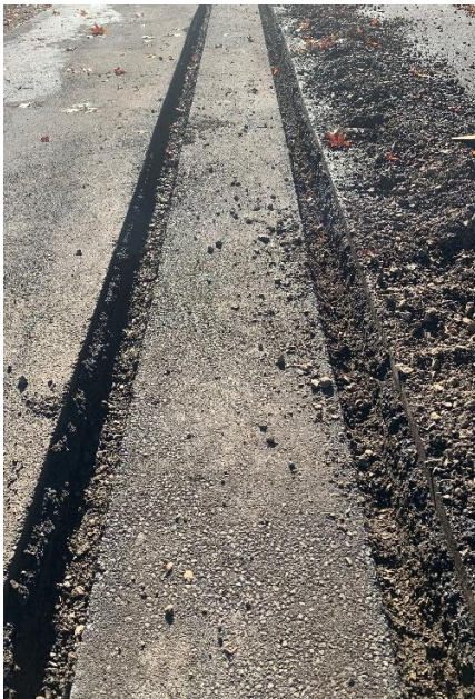
Figure 20. Asphalt Cut Total 23 cm (9 in) depth
