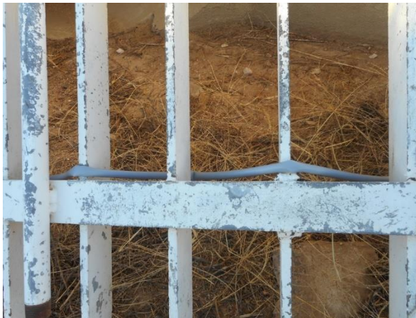
Figure 4: Example of an excessively small bend radius resulting in kinked conduit. This can impact fiber sensitivity and over time will degrade the conduit and fiber.
