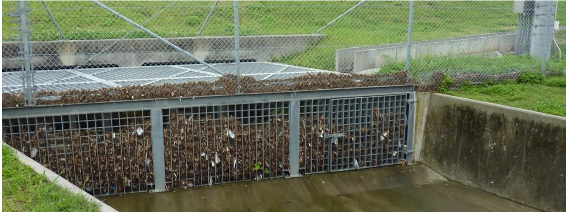
Figure 1: Excess debris in culverts should be removed. The debris may increase the Nuisance Alarm Rate(NAR) and also provides an intruder cover from visual identification.
