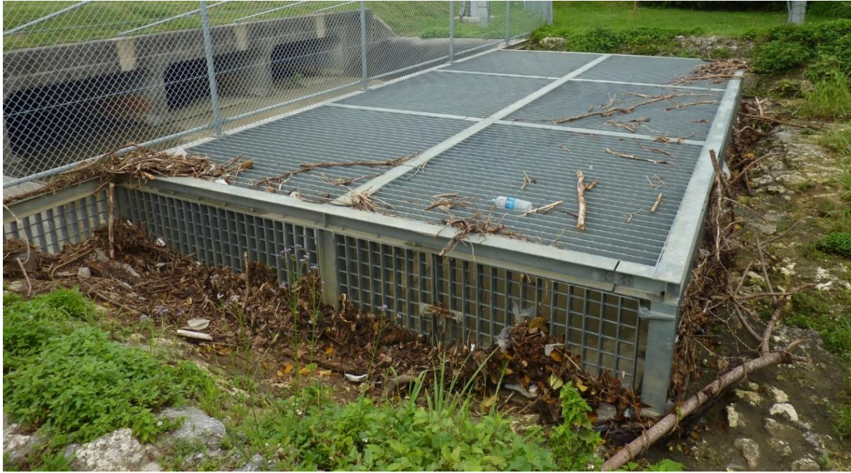
Figure 5: The above culvert requires the sensor to be deployed on all four sides of the grating. For this culvert, weaving would potentially result in kinks in the conduit and would have to be avoided. Installing on the protected side if possible would be preferable when weaving is not an option.
